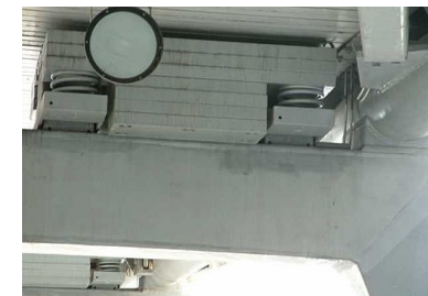
Tuned mass damper
