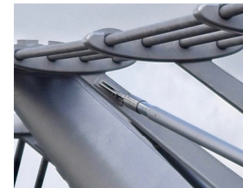
Moving end of pier damper
